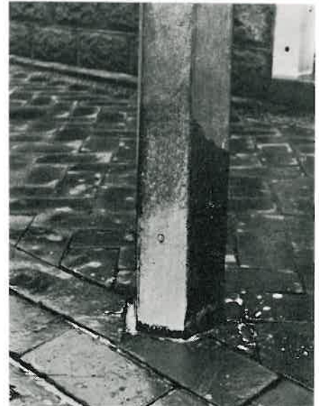
Close-up of a 14-year-old aluminium column before during and after cleaning with soap and water. Note bitumen coating above ground level and potential corrosive water traps around base.
